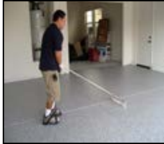
Used as a 1 coat high build sealer over a Flaked Garage Floor
