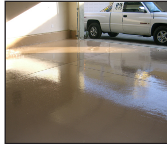
4010 Waterbased Epoxy applied to a garage floor without a clear topcoat
