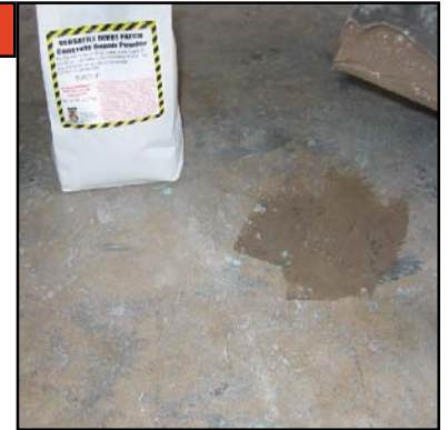
Spalled Concrete filled with DIVOT PATCH
